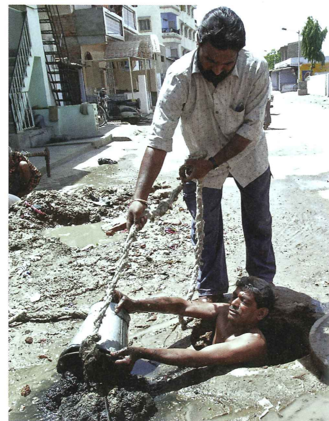
7.27 Dalit workers cleaning a blocked sewer
